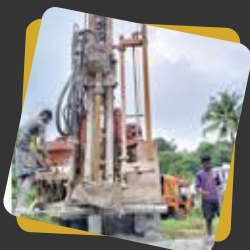
BOREWELL & MOTOR For 1st 100 Ft - Rs.100/- For 2nd 100 Ft - Rs.110/- For 3rd 100 Ft - Rs.120/- For 4th 100 Ft - Rs.130/- 7" pipes - Rs.280/- Feet 10" pipes - Rs.500/- Feet
