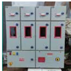
EB PANEL BOARD (Including Cables and Labour)
